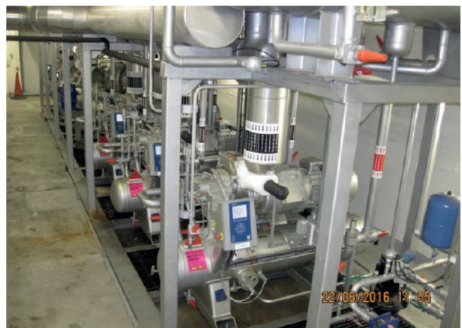
Figure 4: Condenser for the ammonia system.
