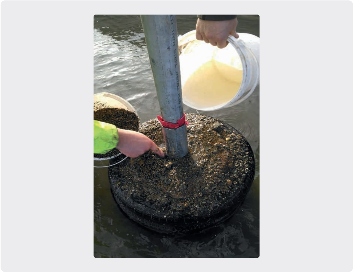
Figure 11: Top of a 3-tyre stack placed over an outer pipe and with an inner pole shimmed in afterwards. Gravel washed down into spaces between pole and hole to tighten the structure. Gravel washed in to hole at each tyre level.
